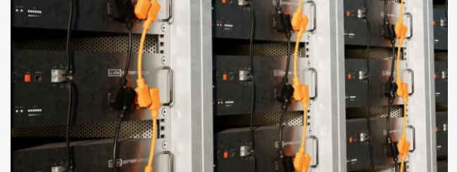
Data Center/Battery Backup Infrastructure
